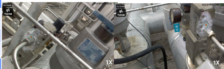
Inspection case of a chemical plant in Henan province —Gas leak
